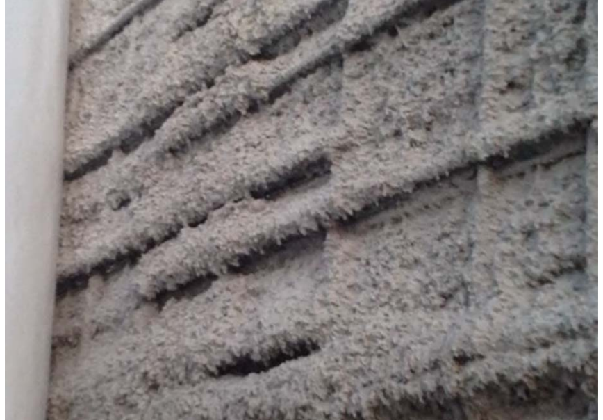
Fig. 5. Visual evidence of buildup on the reinforcement was ignored by the nozzle man. Note the massive voids that have formed behind the bars.
