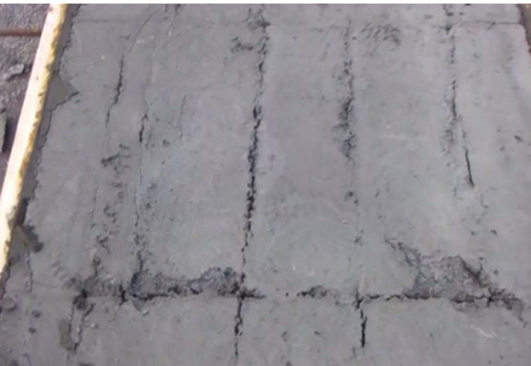
Fig. 6b. Further evidence of tracking visible from the formed side.
