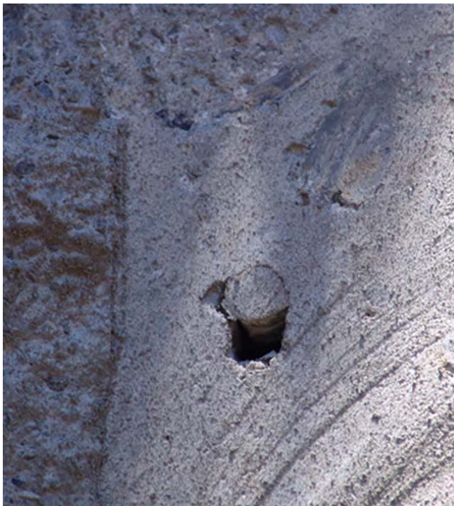
Fig. 4: Void beneath reinforcement in saw cut specimen occurred from downward movement.
